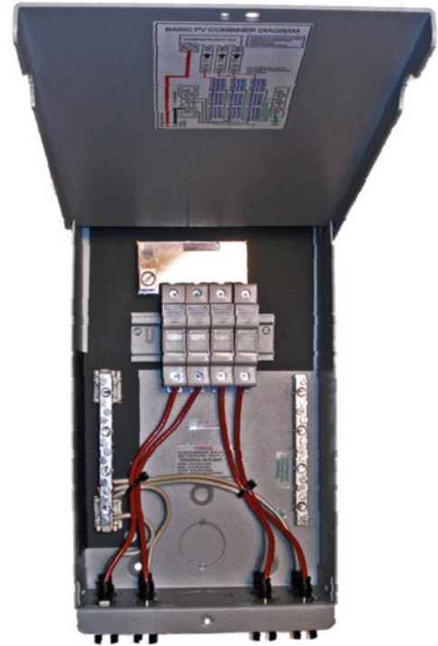
MNPV4 Factory wiring
