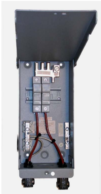
MNPV2 Factory wiring
